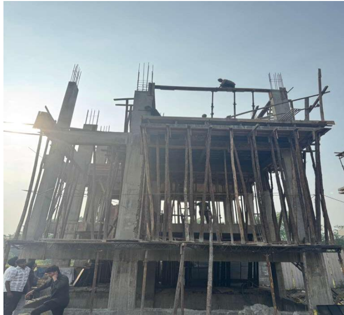
c. Person working at higher level without safety Fig. 4 (a, b, c ) Lack of safety practices
